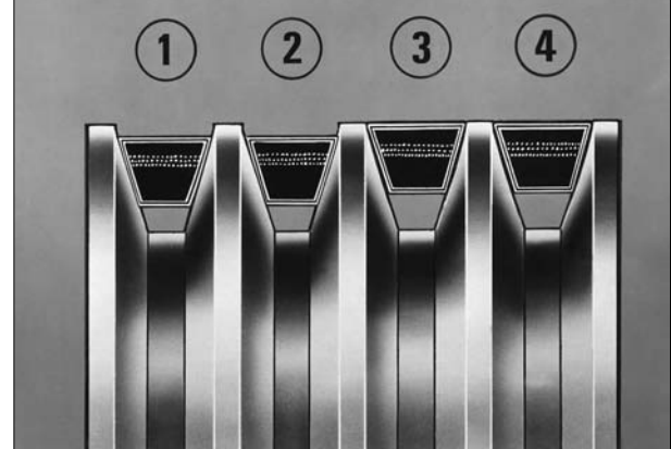
Fig. 7 – Irregular sheave grooves
